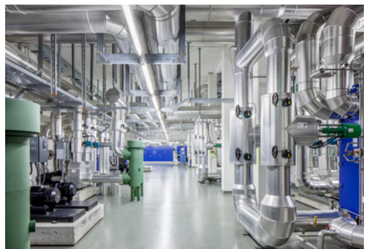
The three floors of the computer building. From bottom to top: resource deck, installation deck, machine room. (Picture: Marco Carocari and CSCS)
