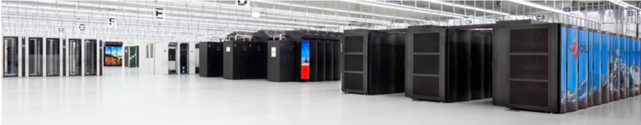
An overview of the machine room. (Picture: CSCS)
