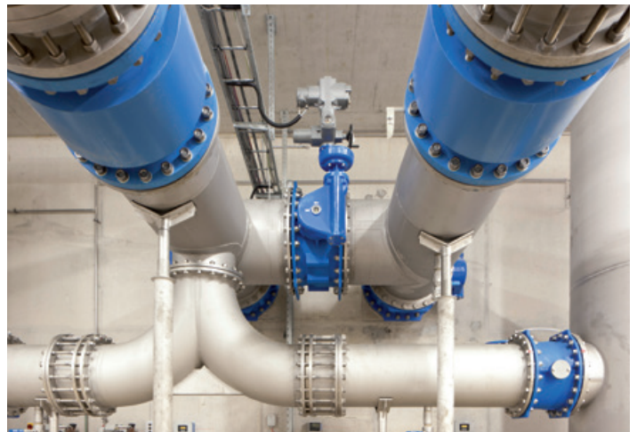
In the labyrinth of the pumping station: five metres beneath the lawns of Parco Ciani, over 700 litres of water per second are pumped out of Lake Lugano. (Picture: Marco Carocari)
